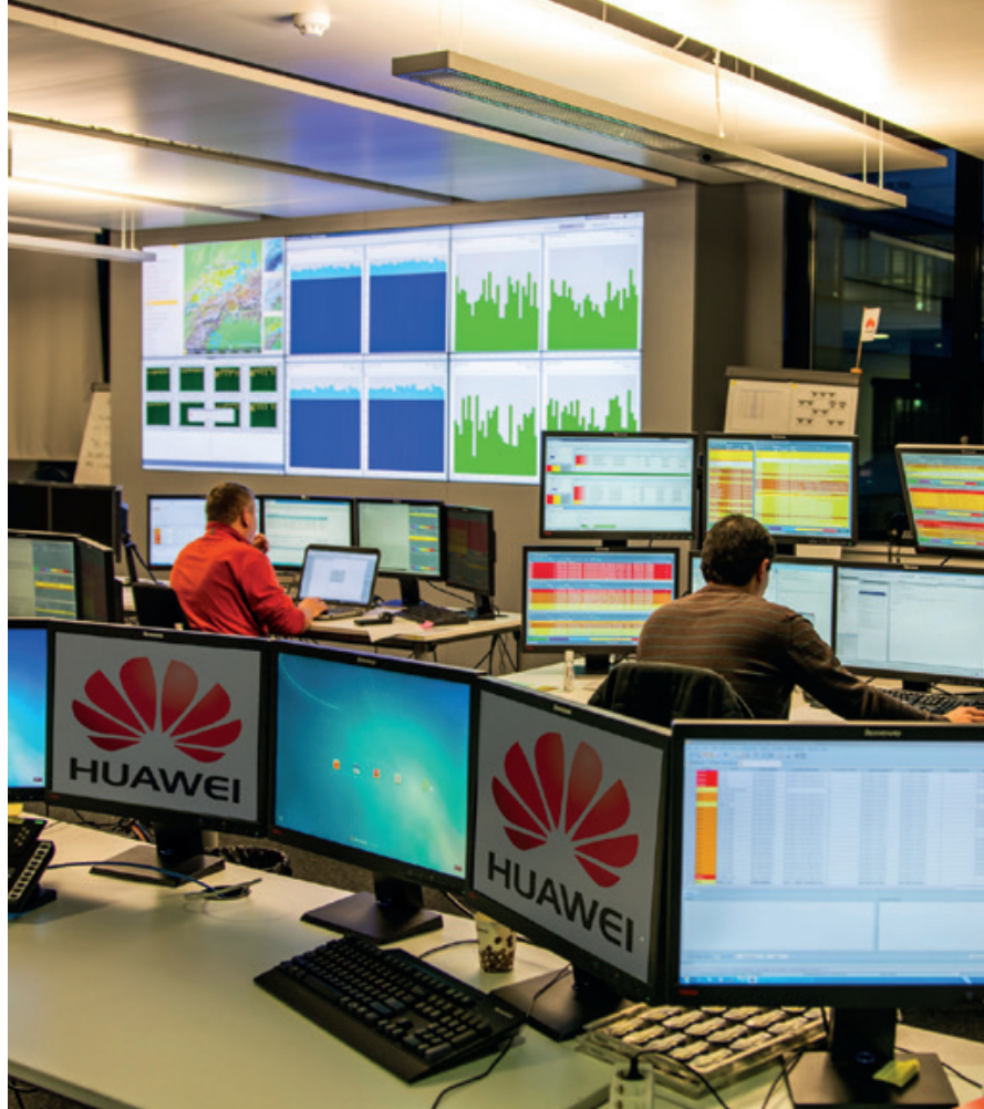
Huawei Network Operation Center
